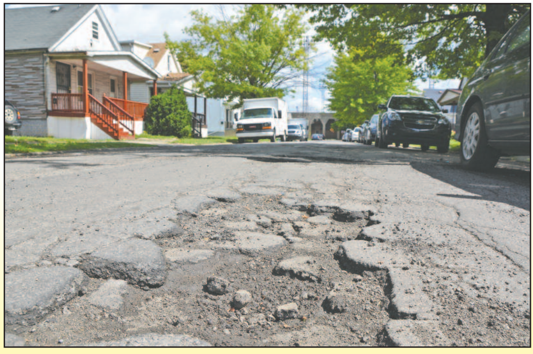
Starting in mid-September, a portion of Goodson near Gallagher will be torn up and repaved. A scaled down repaving project will also occur on Hanley. The work will be paid through a state road fund, and will total over $500,000.
