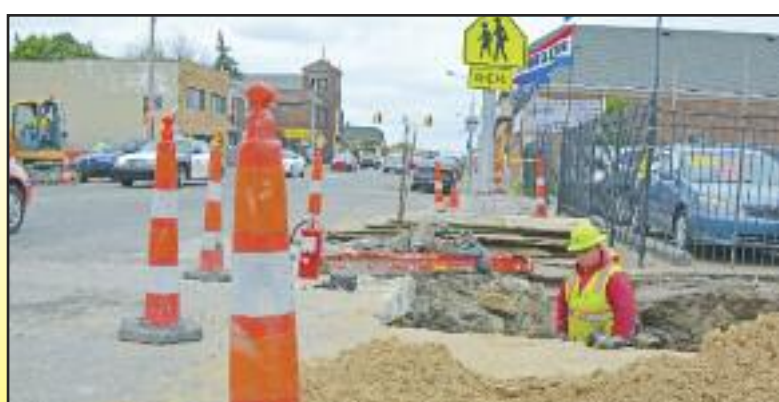
New gas mains are being installed along Conant, which has caused traffic congestion. The work should be completed in two weeks, but there will be more construction work throughout the city in the months to come.
