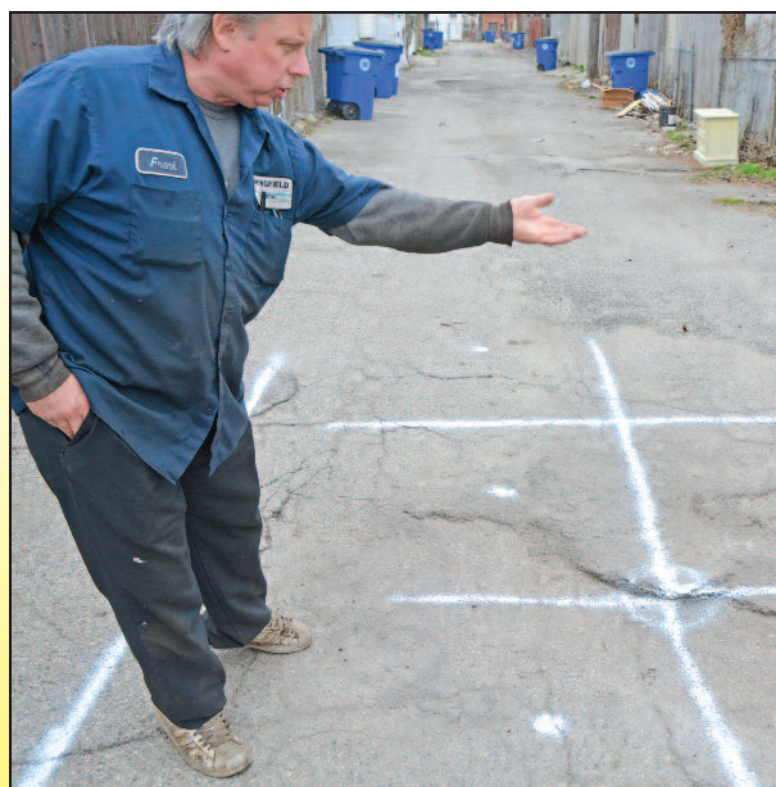
Dave Tulecki points out a sinkhole that formed in the alley behind his Fleming house. The city is now charging homeowners for repairing sinkholes caused by leaking sewer lines.
